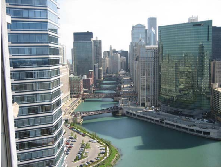
View looking east from the 31 st Floor of the Left Bank Condominiums, a 38-story high-rise under construction adjacent to the Chicago River. Photo taken by Gina Schoengarth, Jr. Architect, Fall 2006.
